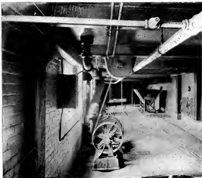
Ashes fall through chutes in the stoking floor to narrow gauge dump cars which are lifted by elevator to ash hopper.
